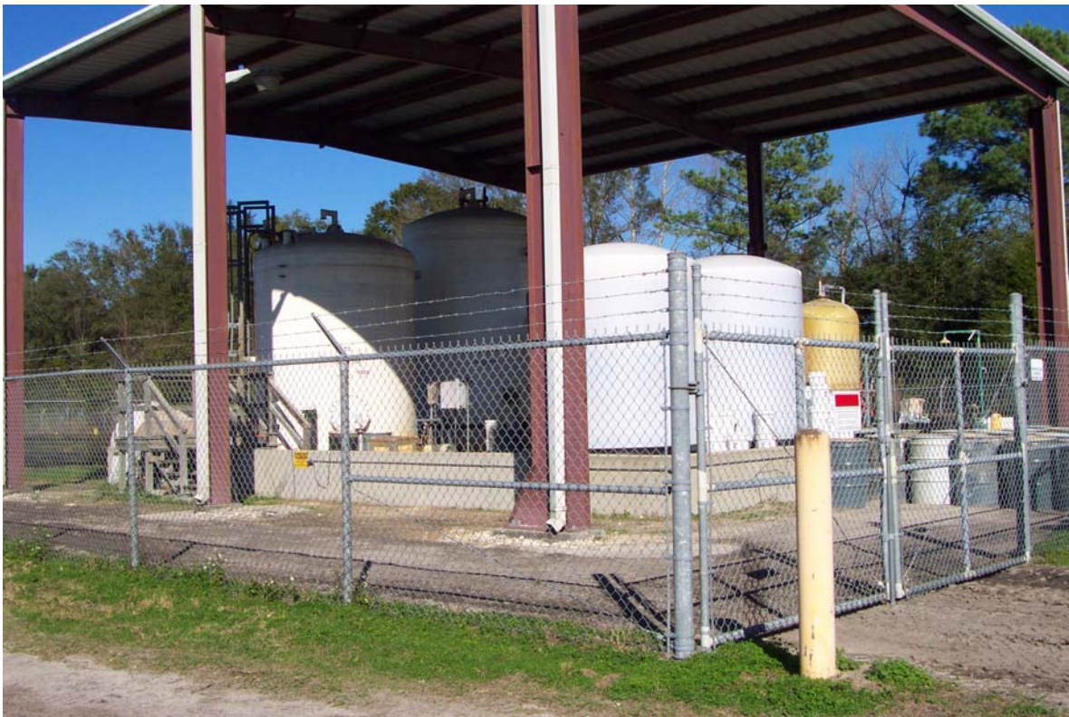
PHOTOGRAPH 7. WATER TREATMENT PLANT, CLOSE-UP, KOPPERS 1 FEB 06
