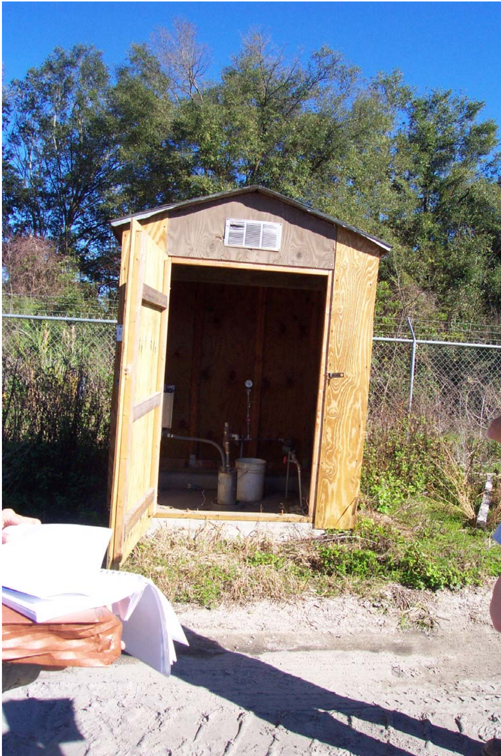
PHOTOGRAPH 4. TYPICAL EXTRACTION WELL AND PUMP HOUSE, KOPPERS, FEB 1 06
