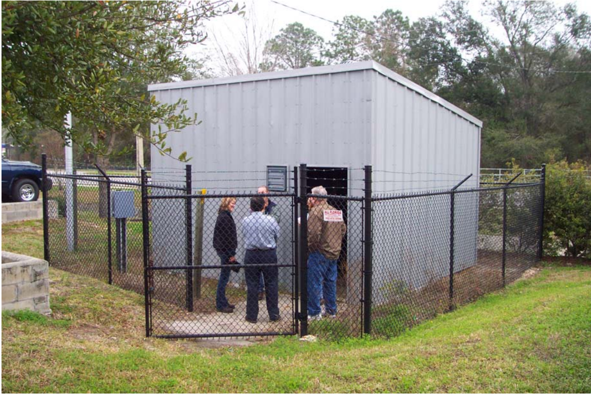
PHOTOGRAPH 18. CABOT LIFT STATION, 2 FEB 06
