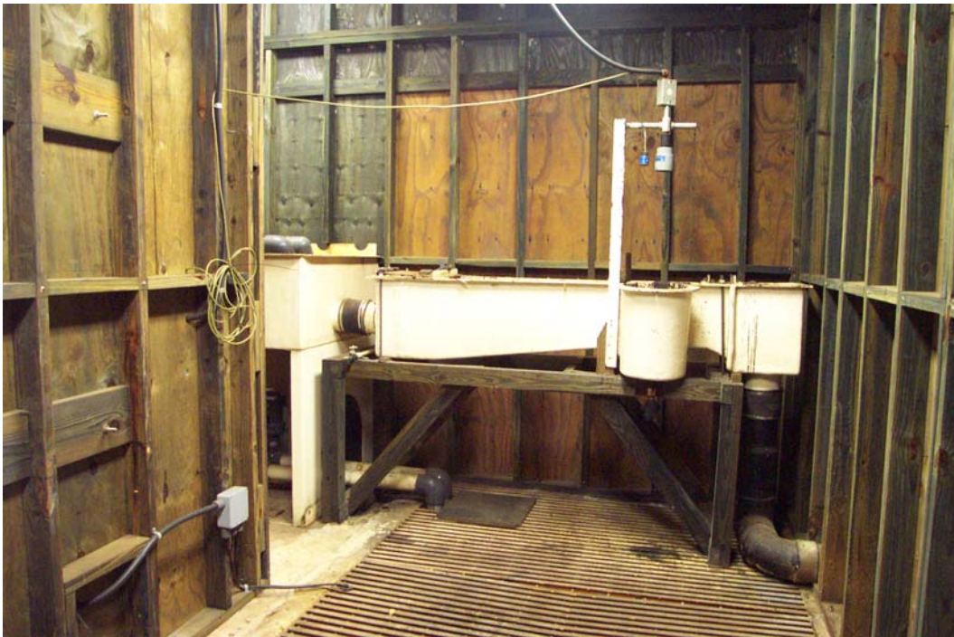
PHOTOGRAPH 19. INSIDE CABOT LIFT STATION, CABOT 2 FEB 06
