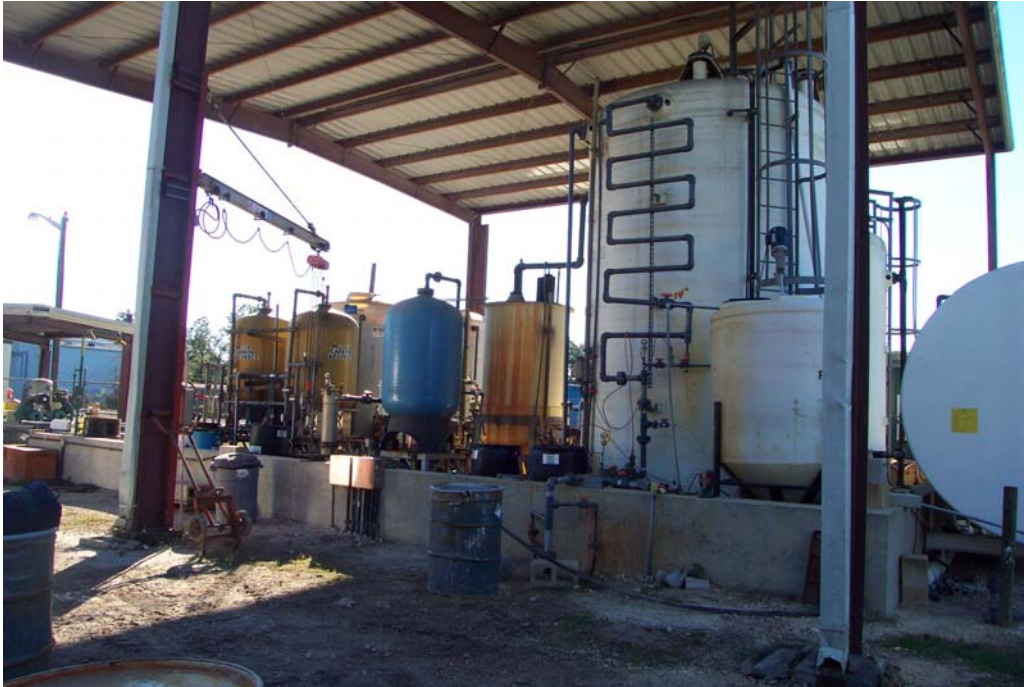
PHOTOGRAPH 8. WATER TREATMENT PLANT, INTERIOR VIEW, KOPPERS, 1 FEB 06
