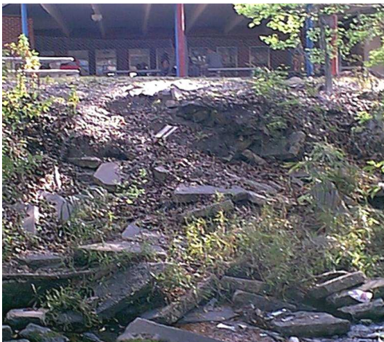
Tumblin Creek bank failure at PK Yonge School
