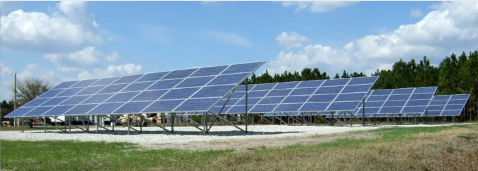
Dec 31, 2008 installation of a 26kW photovoltaic array at the Alachua County Waste Transfer Station
