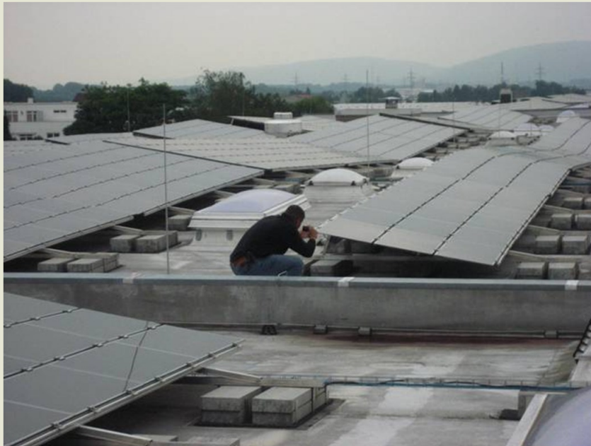
A typical commercial solar roof installation in Germany. Photo by: Ed Regan
