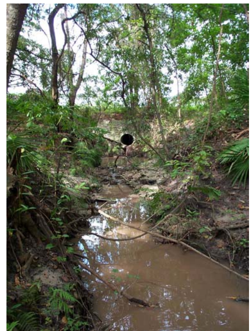
Illicit discharge to Springstead Creek from a stormwater conveyance system south of NW 39 th Avenue (Photo Credit: Joy McBane, Alachua County Environmental Protection Department)
