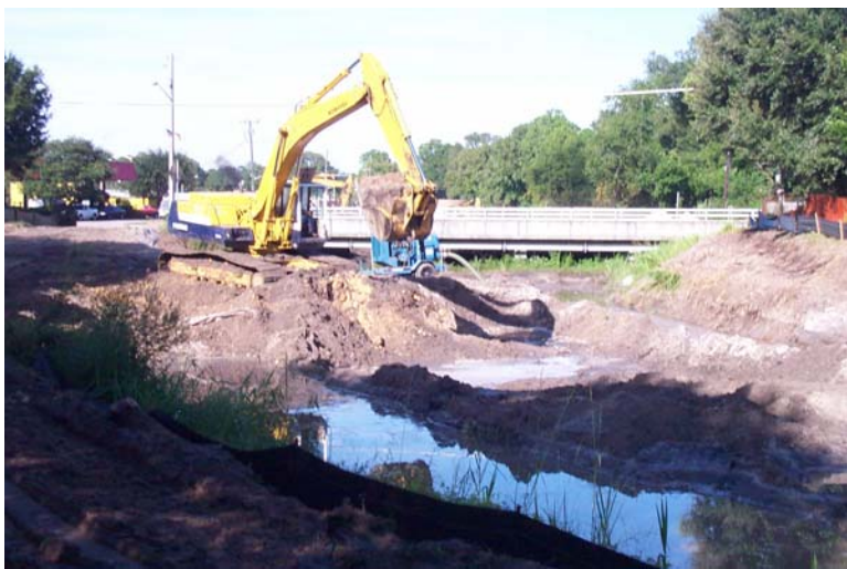
FDOT Sediment Trap construction in Hogtown Creek east of NW 34 th Street (Photo Credit Robin Hallbourg, Alachua County Environmental Protection Department)
