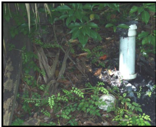
Wastewater Line Cleanout next to Sweetwater Branch
