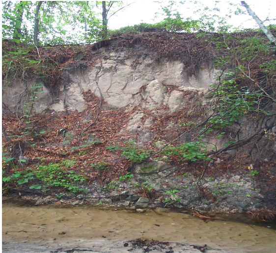
Severely eroded bank along Little Hatchet Creek near the airport
