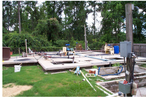
Brittany Estates wastewater treatment package plant
