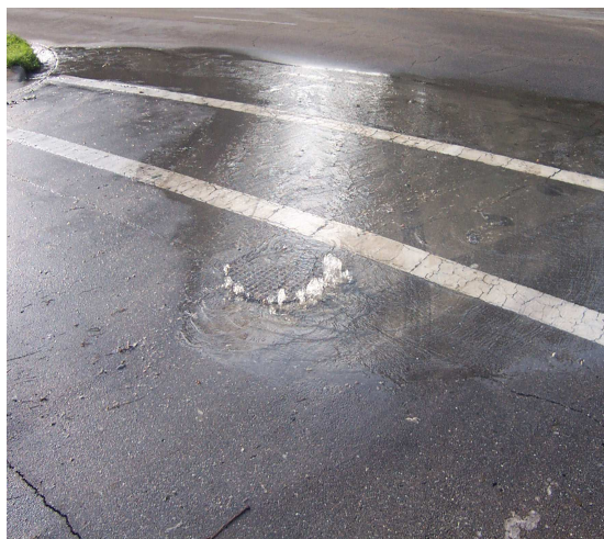
A leaking manhole discharging untreated wastewater to the stormwater system.
