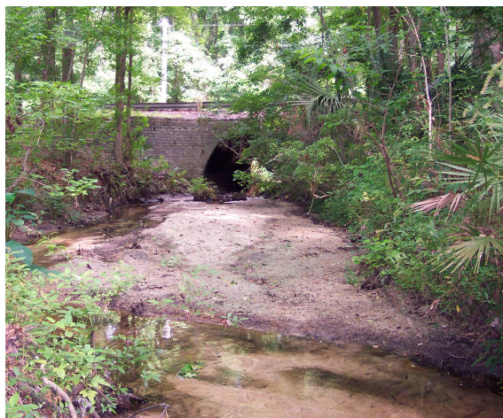
Sand deposited upstream of a culvert in the North branch of Little Hatchet Creek near the Airport.
