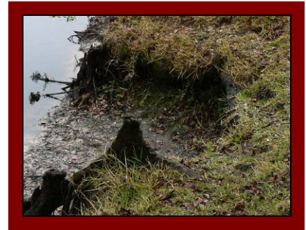
Examples of bank erosion along main spring run
