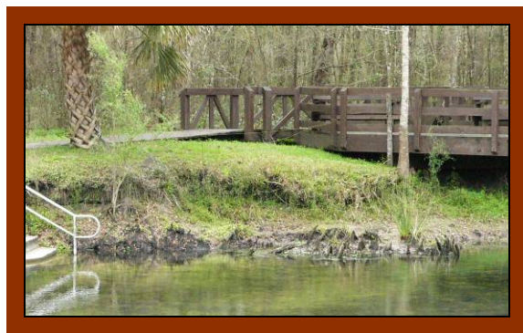
Bank erosion at Poe Spring
