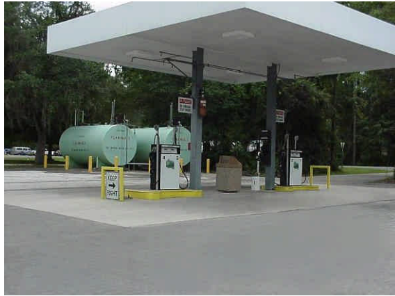
Fleet fuel facility at the Public Works Compound in Hague
