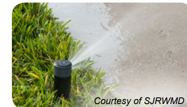
Sprinkler heads that are not adjusted can waste water by spraying onto paved areas.
