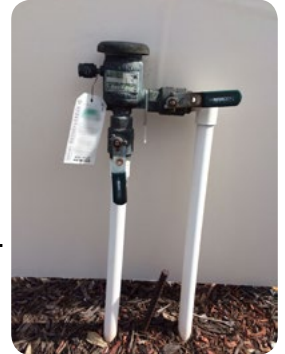
A backflow preventer and regular testing are required by law to prevent irrigation water from flowing back into our drinking water.
