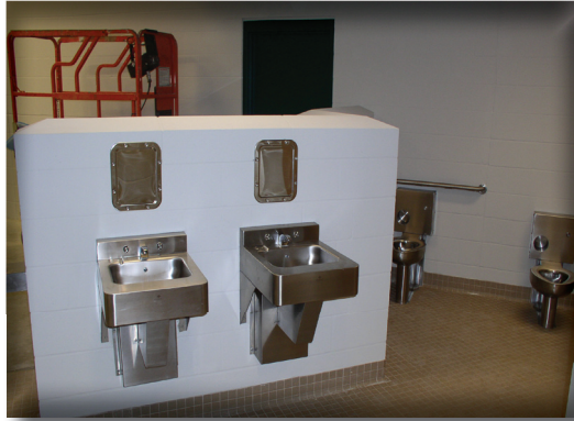
Efficient fixtures at the Alachua County Jail
